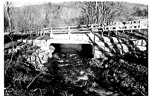
Top: Photo shows the original culvert on County Route 2 prior to replacement. Bottom: Photo shows the replacement box culvert after construction.
