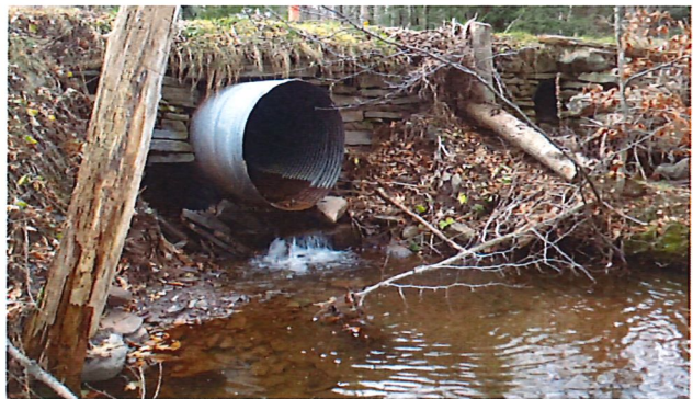
An example of a perched culvert.
